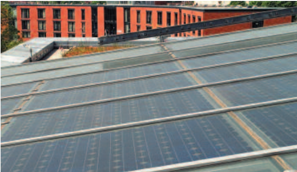
Pic: Jubilee Campus, Nottingham. Photovoltaics can help to reduce a building's electricity demand.
